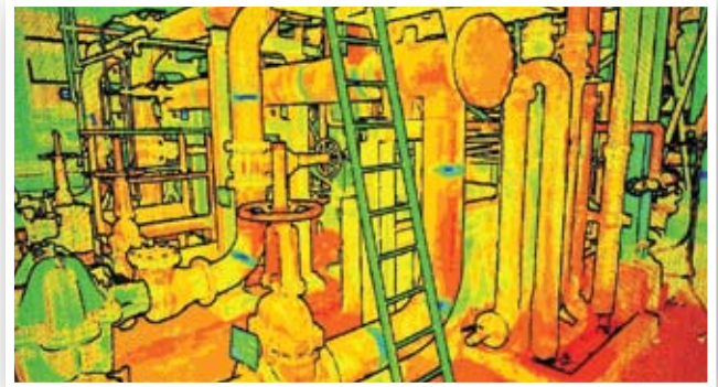
Above: High-resolution 3D point cloud from one of AAM's terrestrial laser scanners.
